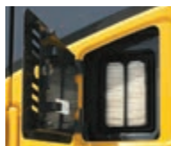
External air conditioner filter
